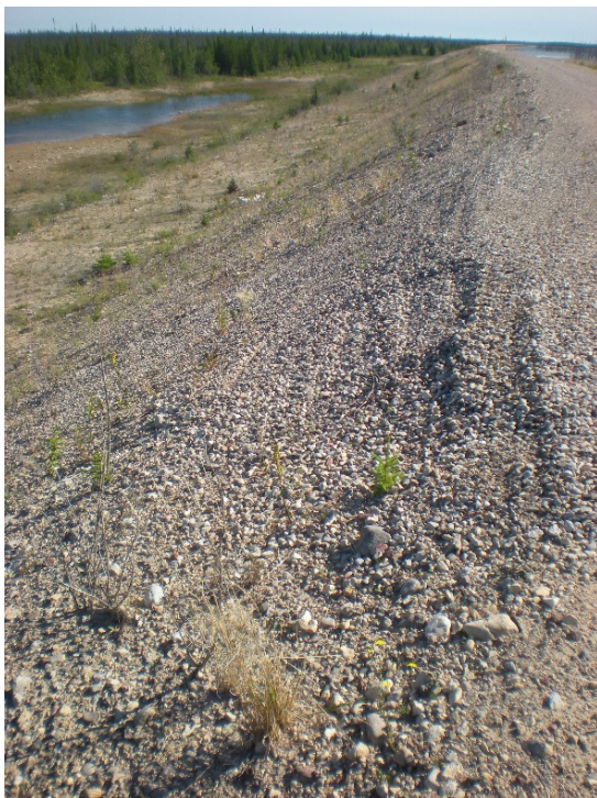
Photograph 8: North Dyke – Downstream Slope (left side of photo) with 2016 Patch on Erosion Feature in Place, Looking East. 27 July 2017
