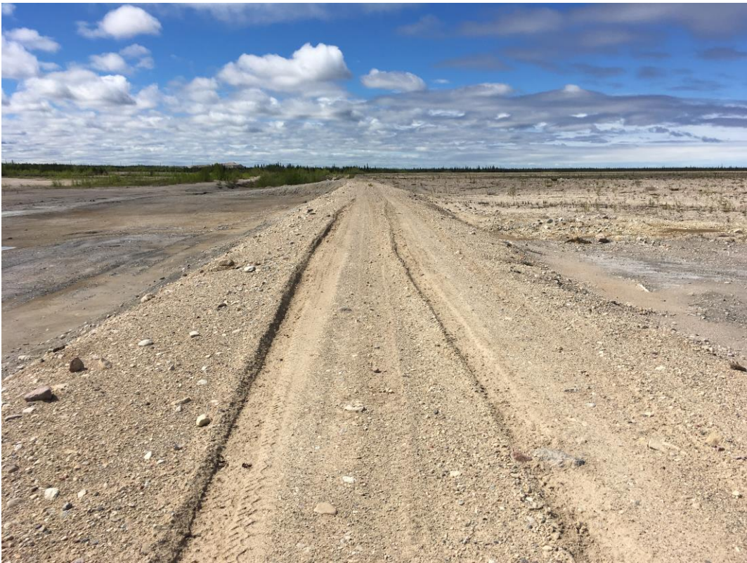
South Dyke, Central area facing east, minor vehicle rutting
