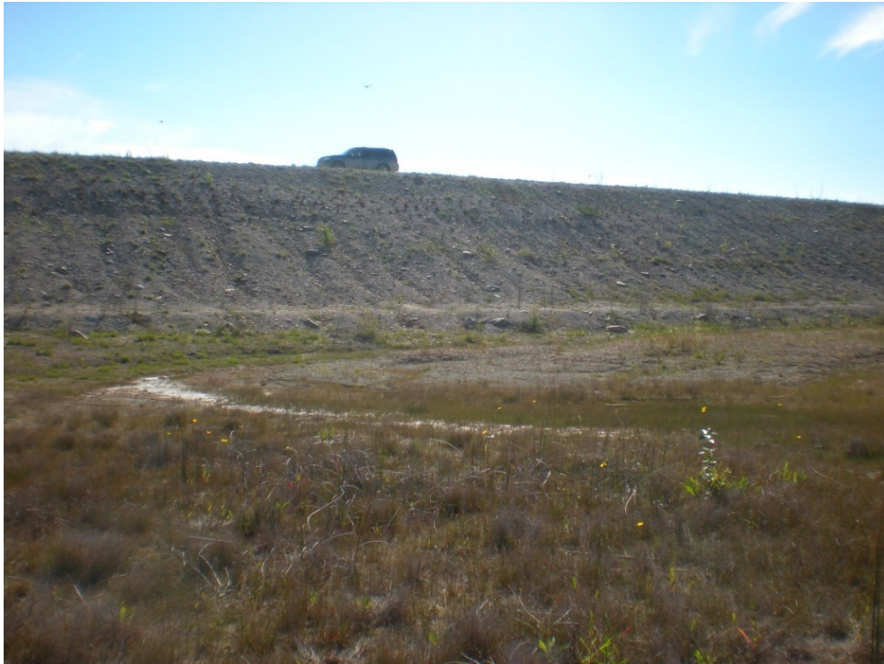
Photograph 7: West Dyke, Downstream Side – Looking East, Stable Erosion Features. 27 July 2017
