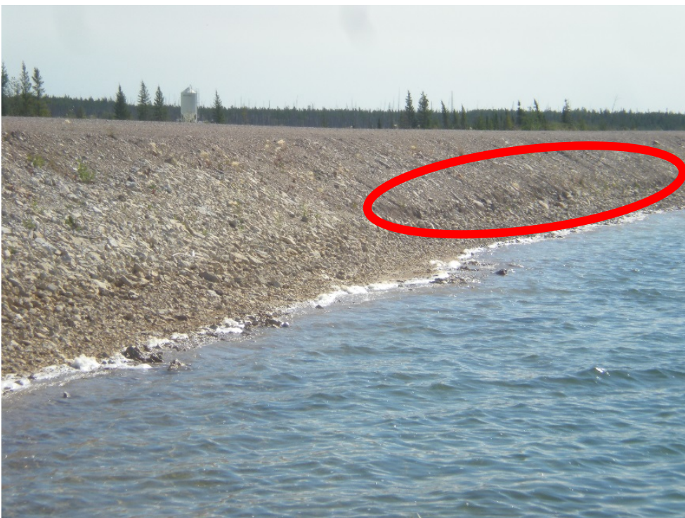
Photograph 10c: North Dyke Upstream Face, Gravel and Cobbles at Pond Waterline, at Dogleg Looking East. Detail Showing Possible Sloughing of Previous Repair. 27 July 2017
