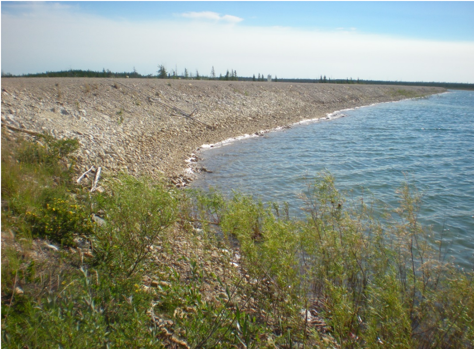
Photograph 10b: North Dyke Upstream Face, Gravel and Cobbles at Pond Waterline, at Dogleg Looking East. 27 July 2017
