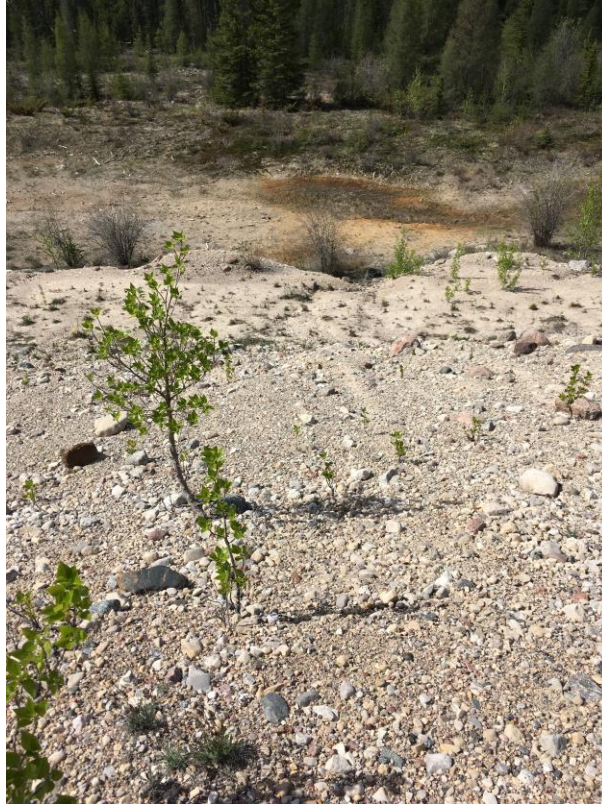
West Dyke, minor staining near toe, Approximate Station 19+00
