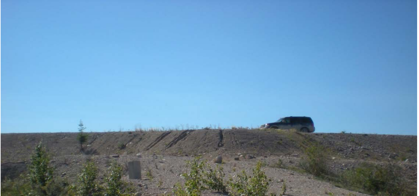
Photograph 9: North Dyke – Erosion Feature on Downstream Slope (former ramp, non-structural), Near Center (dogleg), Looking South. 27 July 2017
