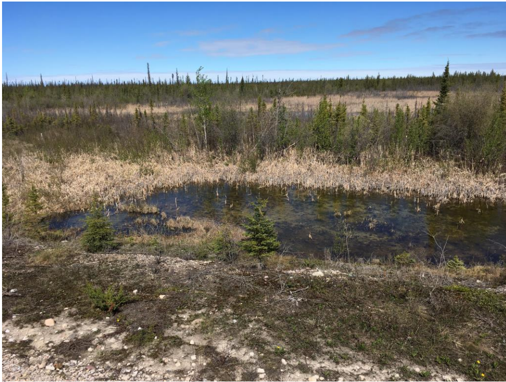
North Dyke, dog leg section, facing north, staining at toe.
