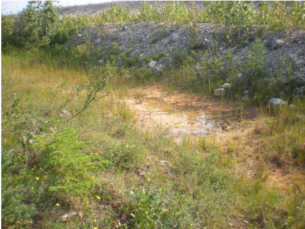
Photograph 5: West Dyke, South End. Ponded Water Downstream Of Toe, Looking North. 27 July 2017
