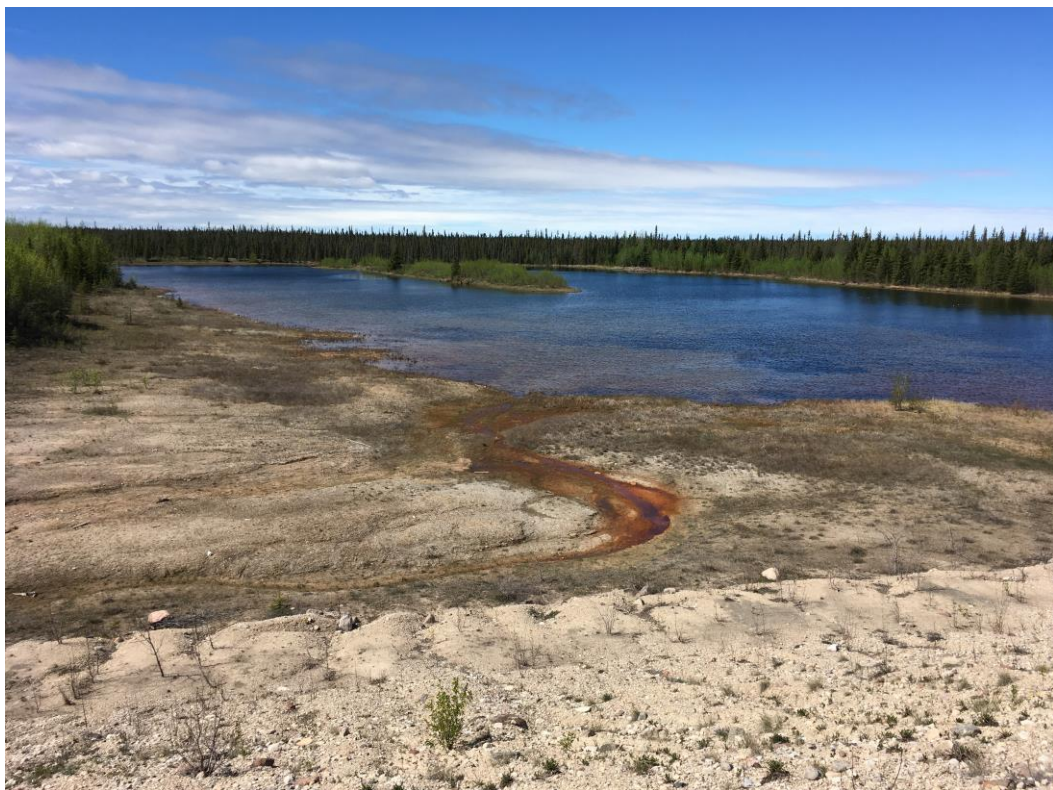
West Dyke, staining near toe.
