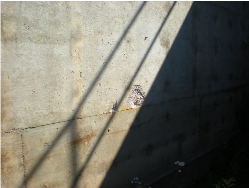
Photograph 11b: Main Pond Spillway (Spillway No. 1). Detail of Limited Spalling 27 July 2017
