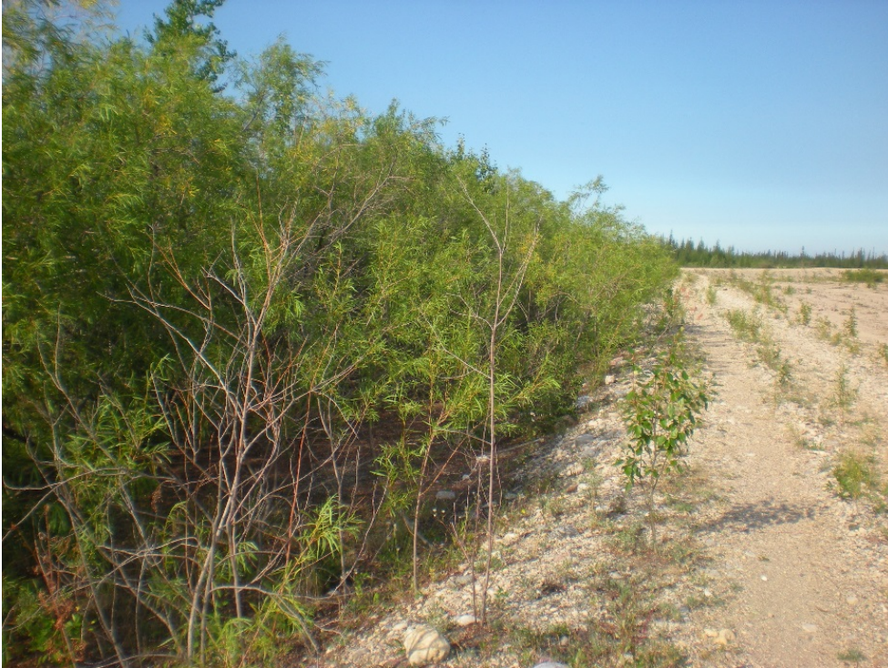
Photograph 3: South Dyke – Downstream Face of West End with Vegetation, Looking West. 27 July 2017
